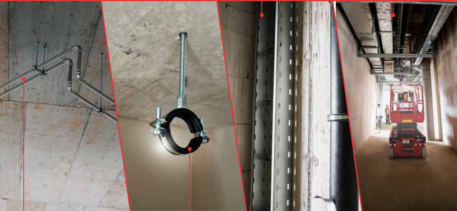
Fastening of piping
